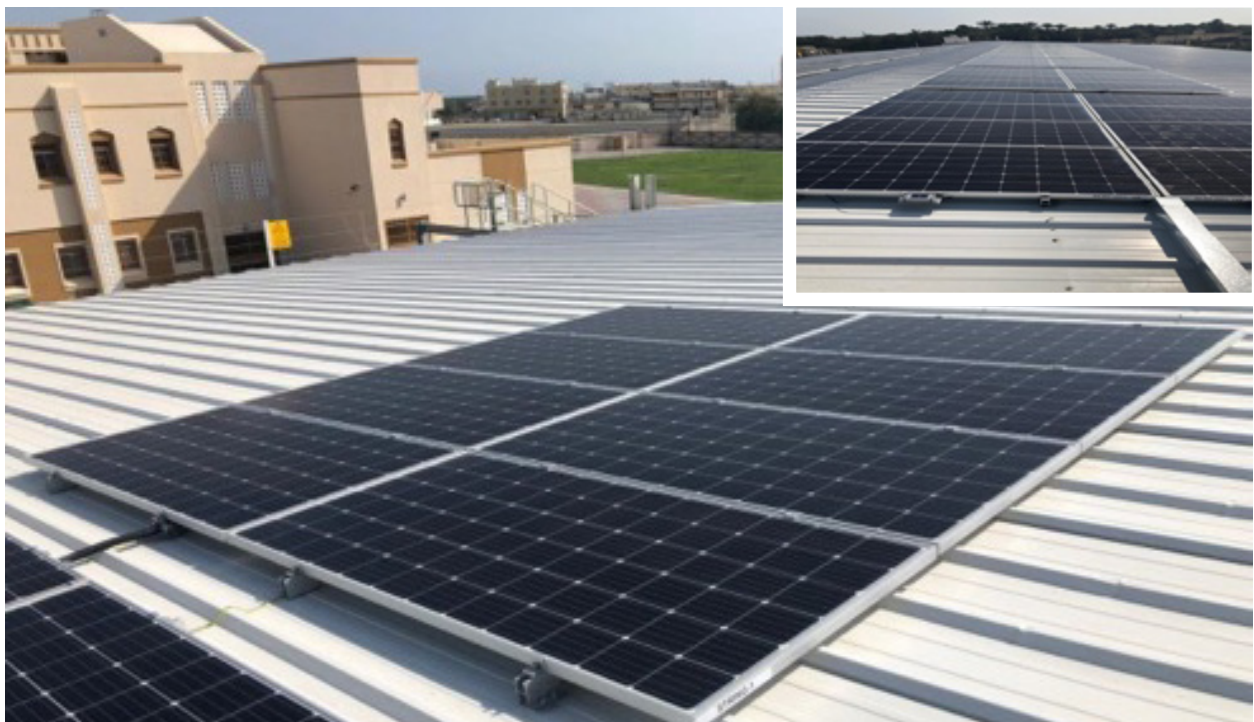
Picture of roof-top PV solar project installed at the school at Liwa.
