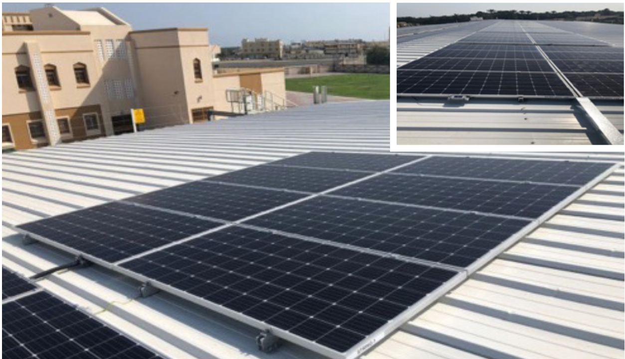
Picture of roof-top PV solar project installed at the school at Liwa.
